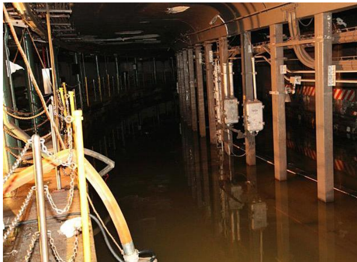
Figure 1 Flooding in New York Subway following Hurricane Sandy (Donohu, 2012)
