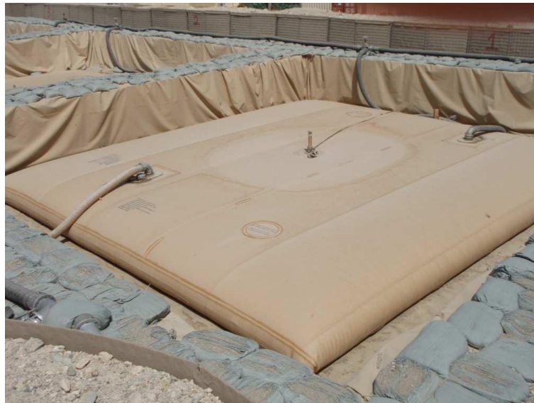
Figure 2: Emergency wet well
